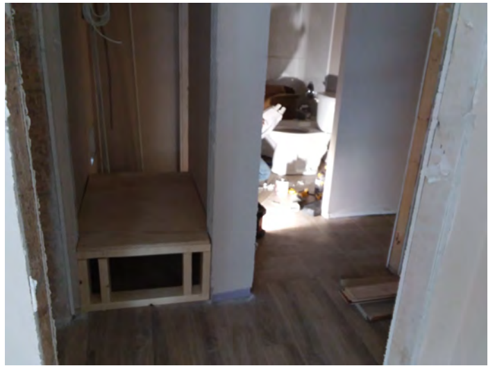
Building 8 C Unit Mech Closet & Hallway
